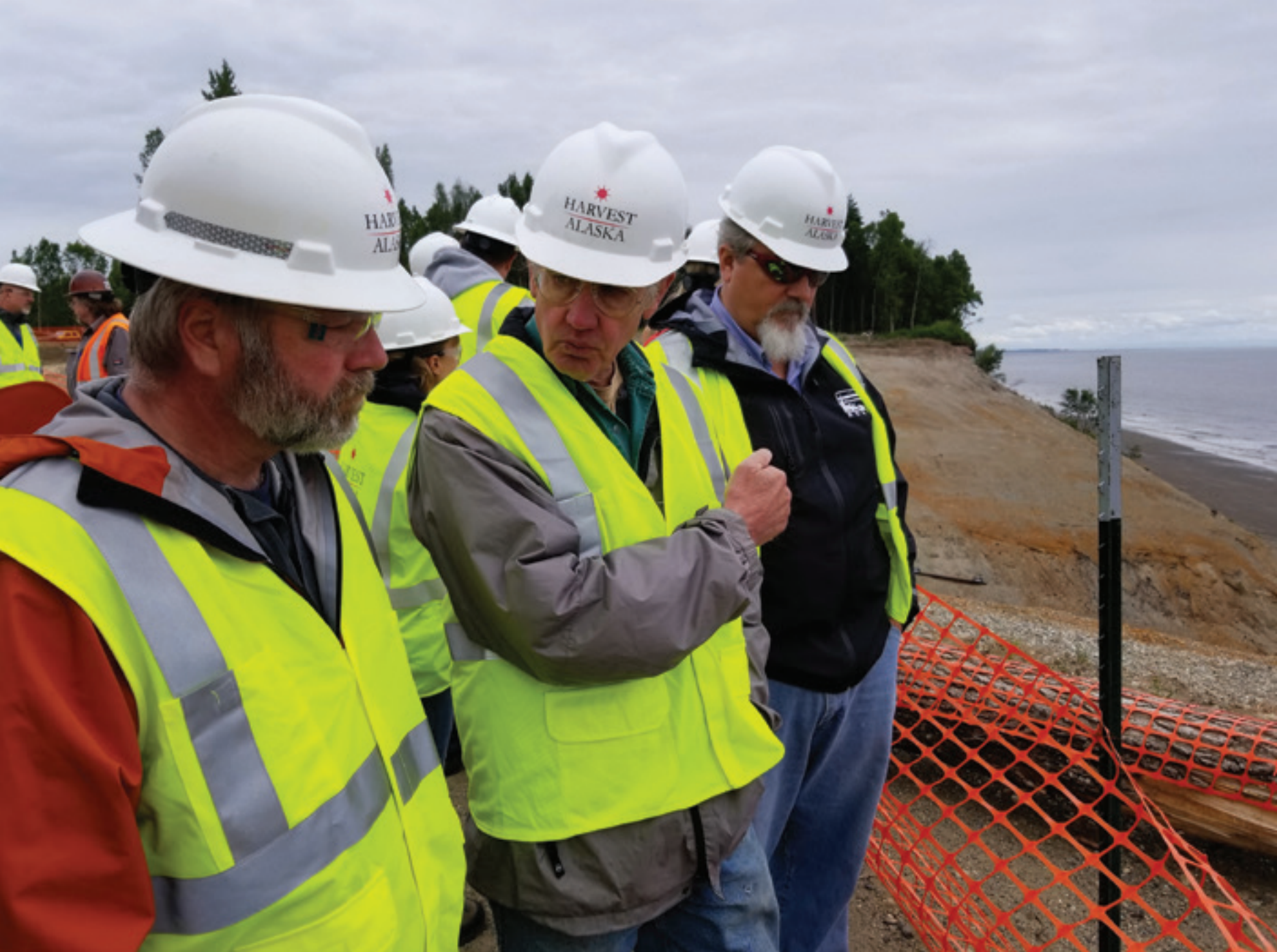
Touring the Cross-Inlet Pipeline installation site at Beluga, from left: Glenn Faulkner (Harvest/Hilcorp), Walt Sonen, (City of Seldovia Representative) and Steve "Vinnie" Catalano (CIRCAC Director of Operations). (Photo: J. Rombach)
